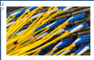
Fibre Optic & Data Structured Cabling System
